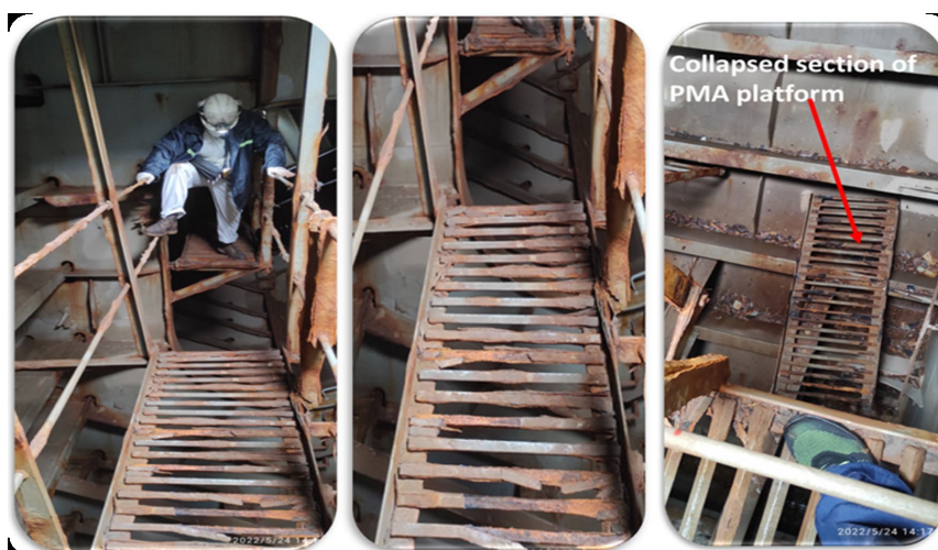
Figure 1: The collapse of the PMA platform during inspections on a 10-year-old bulk carrier
