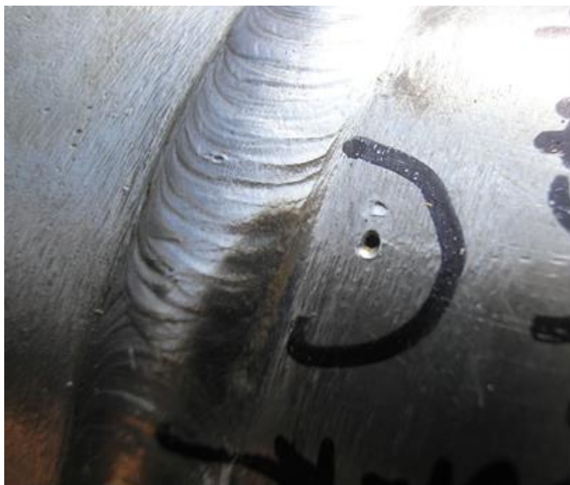
Figure 1 – Example of pitting on cargo piping
